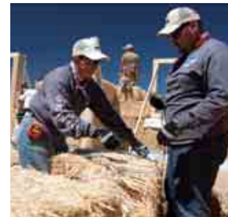
Faye and Gabriel work on customizing bales for window frames and corners.
