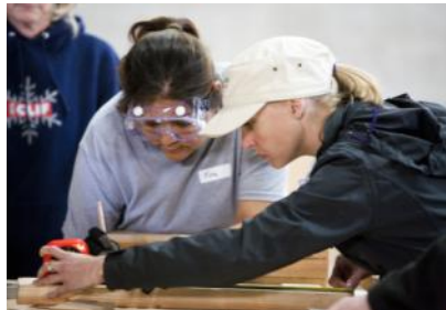
Christina helps measure and cut the wood needed to build the chicken coops.
